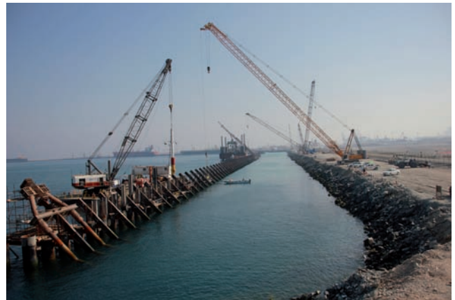
Fujairah's MV piling project under construction and one of the test installations on the left.
